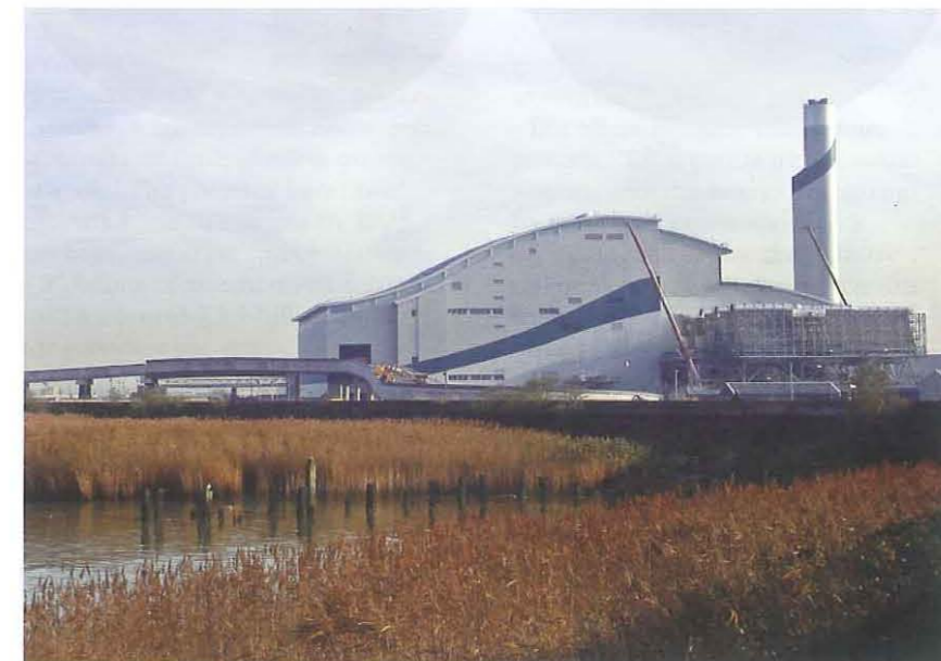
The last of its kind? The under-construction Belvedere incinerator plant in Bexley
